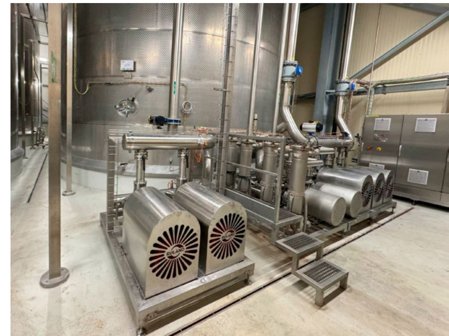
➤ The distribution pumps transport the recycled water from the buffer tank to the liquid production area.
